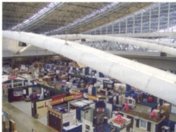
The David L. Lawrence Convention Center is the first major convention facility to use fabric duct.
