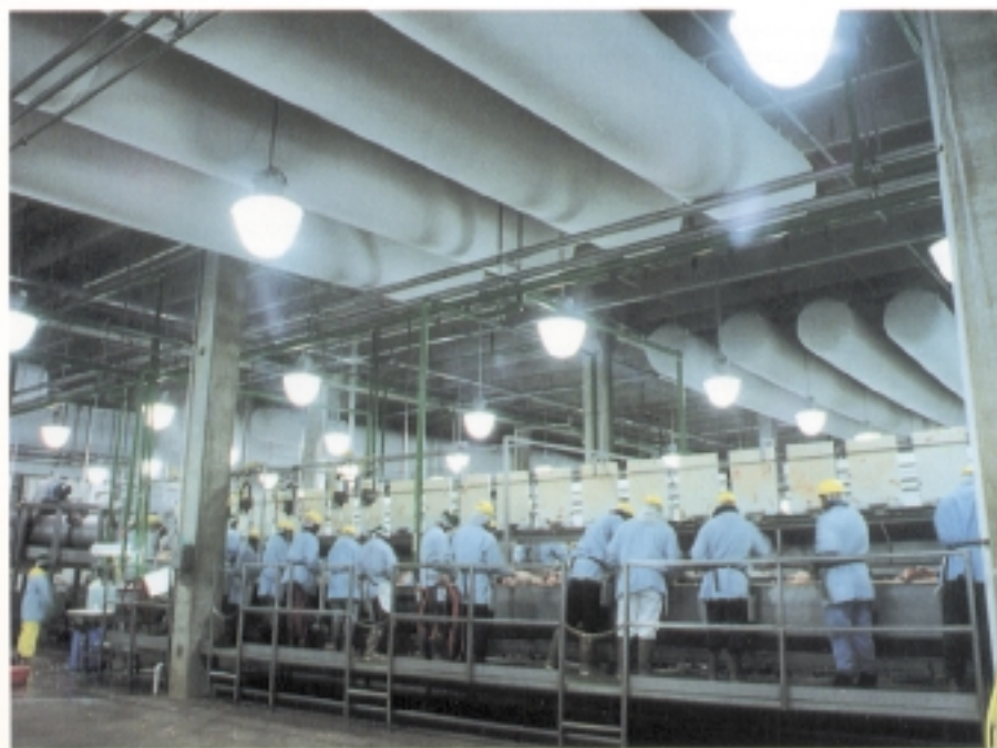
Cool air is evenly dispersed through Ductsox™ fabric ducts, providing a draft-free, comfortable working environment in Carolina Processing's ham boning room.
