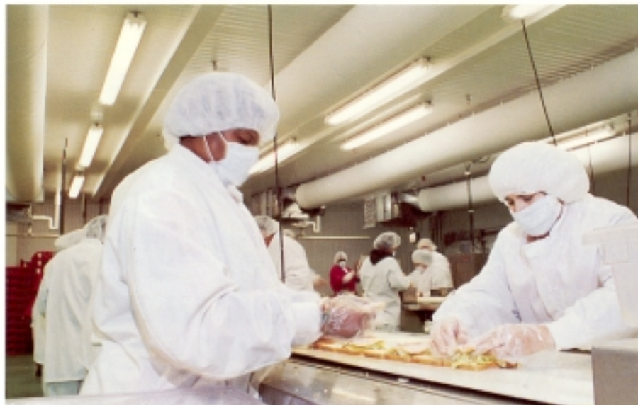
By effectively controlling bone-chilling drafts and the accompanying "wind-chill" effect, DuctSox improve employee comfort, morale and productivity.
